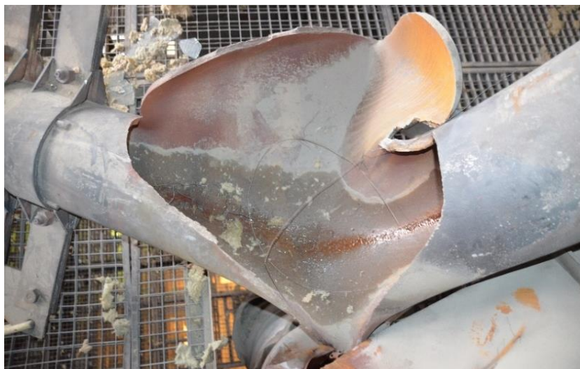
Figure 2 Damaged part of the pipeline bend
