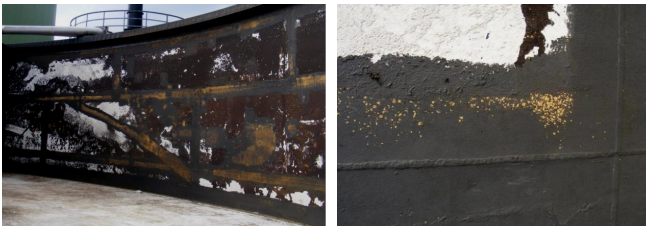
Figure 3 The paint failure after 3 years of service
