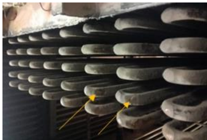
Figure 2 Shot on the bottom of the economizer tubes with visible external wear (indicated by an arrow)
