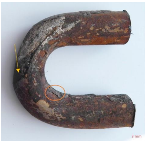
Figure 3 Lower tube bend with a strong abrasive effect of the flue gas
