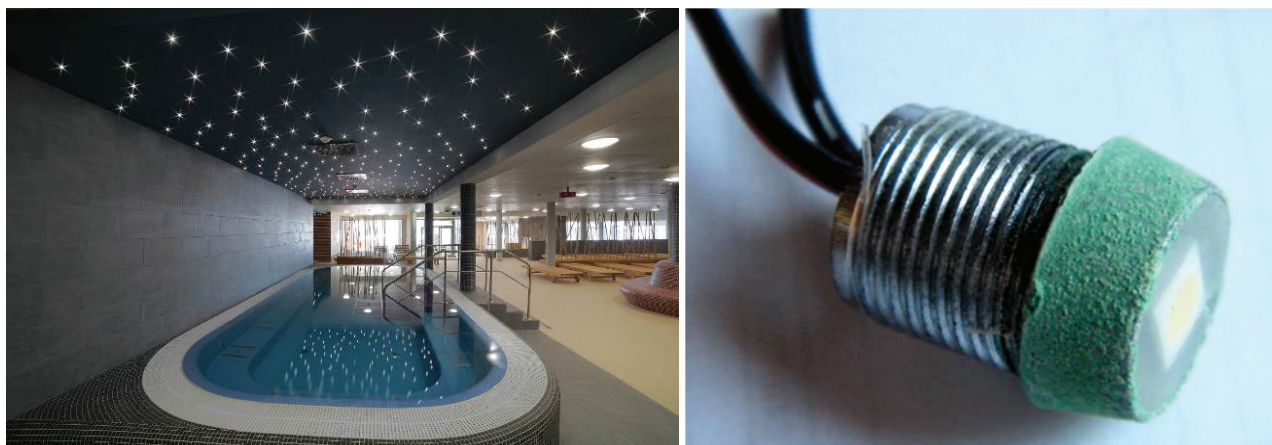
Fig. 5 LED diode lighting of swimming pool and the their corrosion after 1.5 years of service
